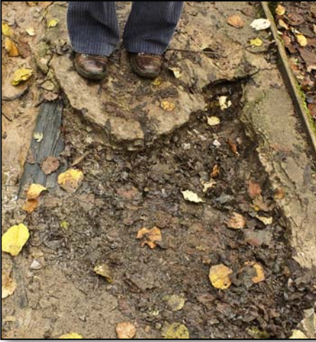
Above: path surface broken and missing, with the membrane visible Right: thick canopy reduces light and prevents new growth at ground level
